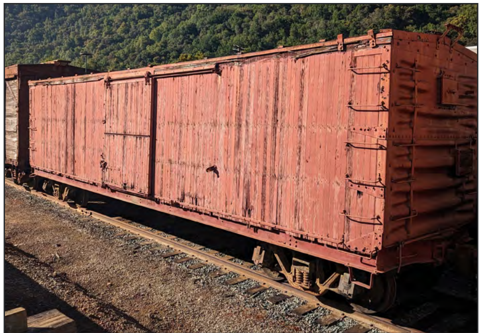
SN 2302 today as it looks sitting at Brightside. It is starting to show age from the weather.
