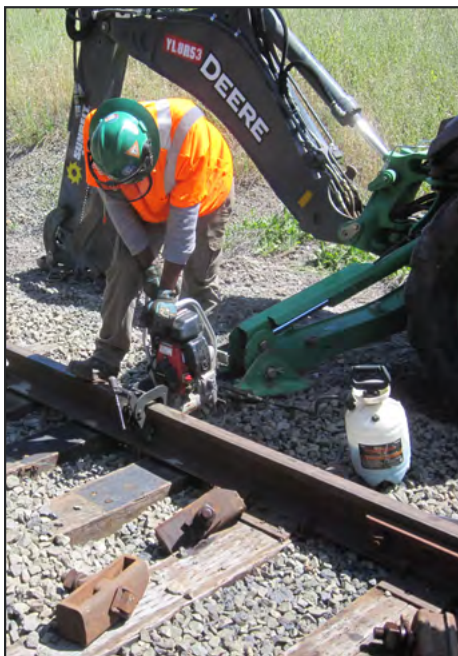
Michael Strider photograph RailWorks crew drilling block holes on running rail for stock guardrail.
